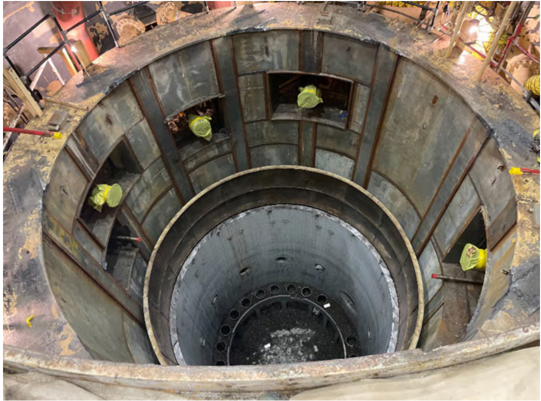
Looking down into the emptied Vermont Yankee reactor vessel with half of it segmented and removed.
